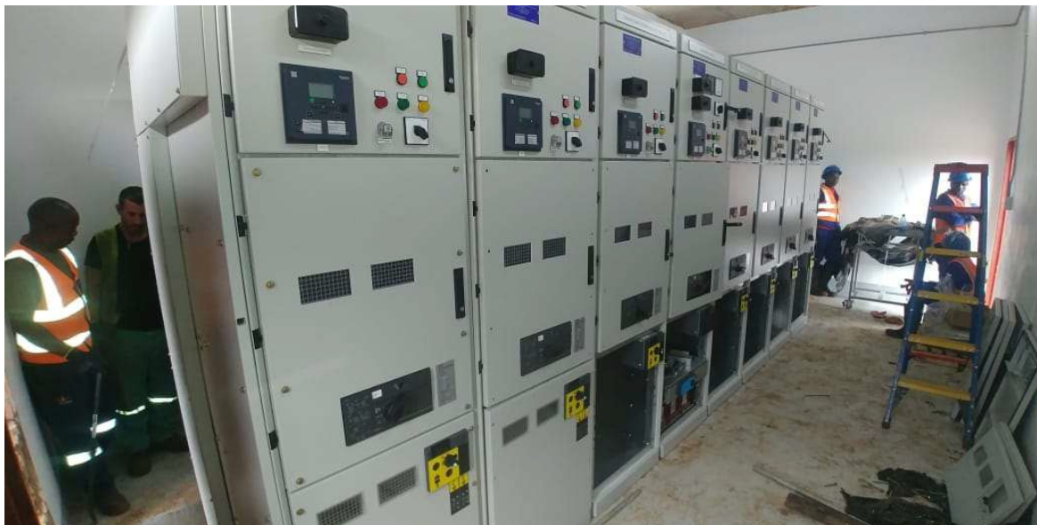
MV (22kV/6,6kV) SUBSTATION, FOUNDRY PROJECT, SPRINGS, RSA
