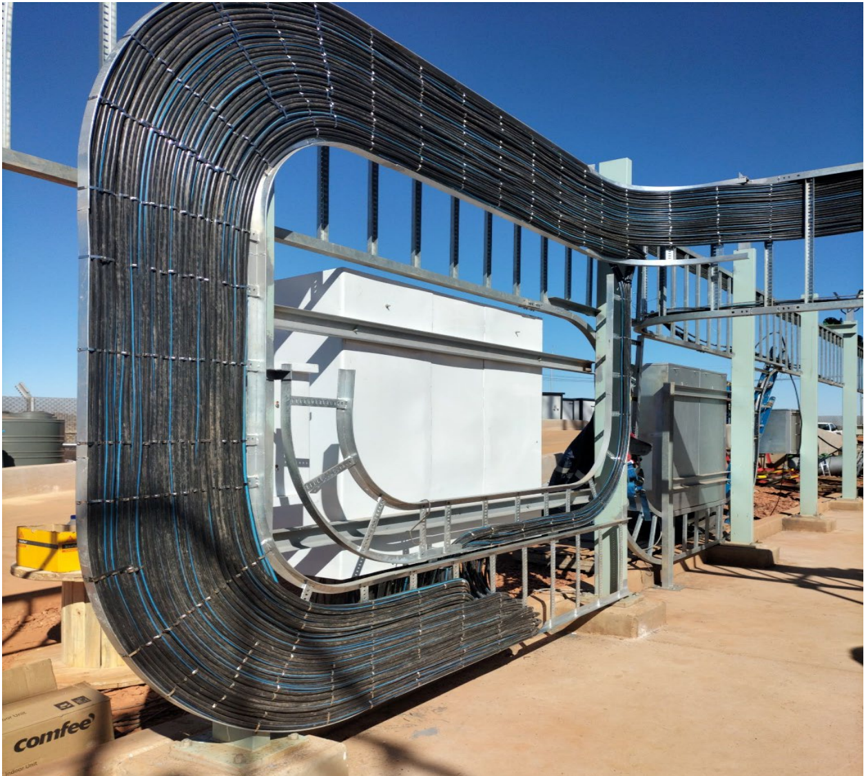
CABLES AND RACKING TO REMOTE PANEL
