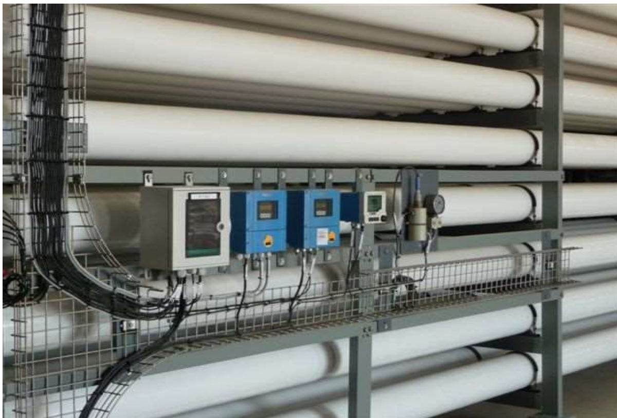
INSTRUMENTATION AT REVERSE OSMOSIS WATER TREATMENT PLANT – NORTH MARA, TANZANIA.
